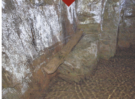
Some way in there is a bend in this long adit and a ledge where a boy may sit, manoeuvring the skips round the corner
